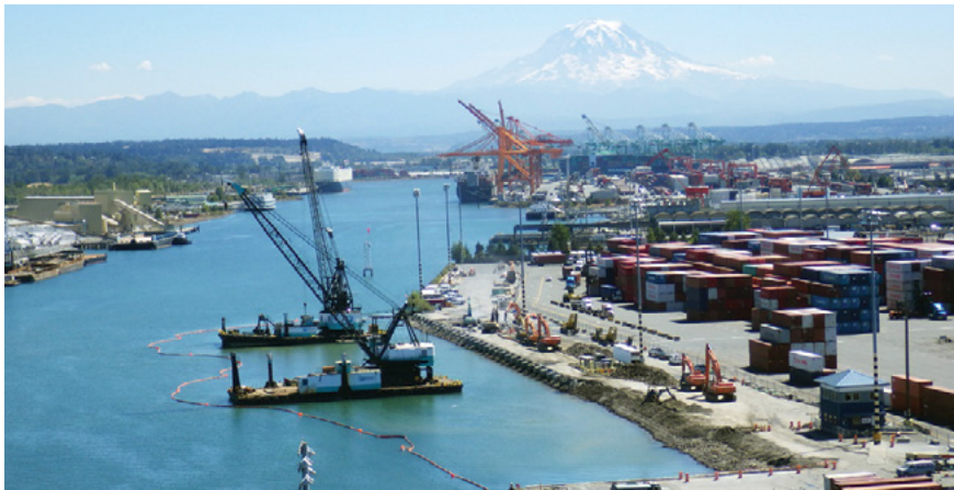
Pile driving to align Pier 4 with an adjacent pier at the Port of Tacoma was limited to certain daytime hours to minimize the nuisance to the surrounding community.
