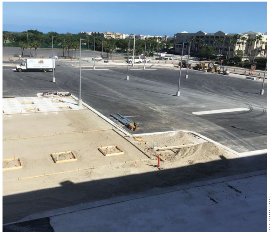
An additional $4.6 million was invested into the stormwater collection/treatment system to create an underground stormwater vault to preserve surface area for parking.
